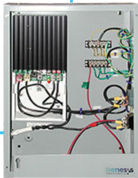
Junction Box with Voltage Regulator
